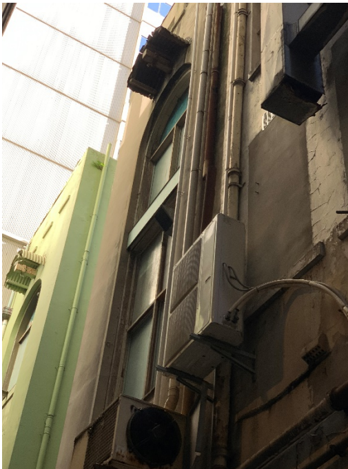
21 Detail view of rear of 15-17 Hunter Street showing arched openings, corrugated iron hoods over hoist and window detailing
